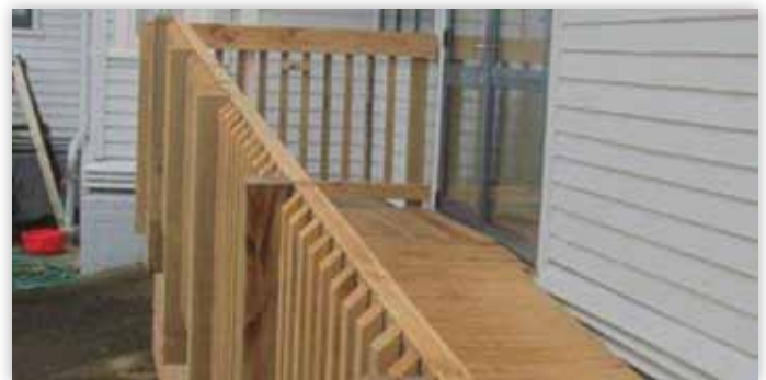
This walkway connecting the two buildings is about to be covered from the rain
