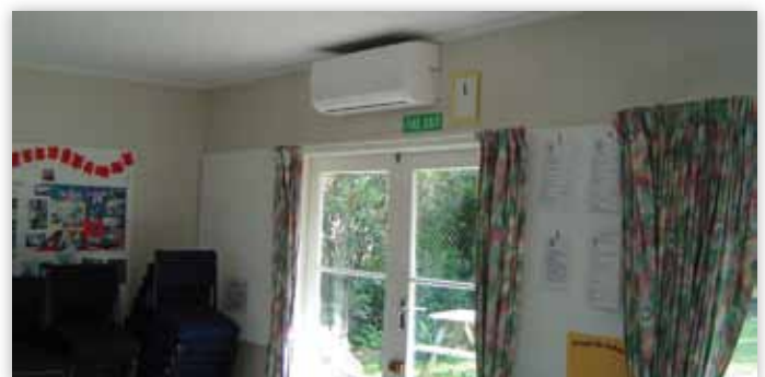
Heat pumps have been installed in three rooms
